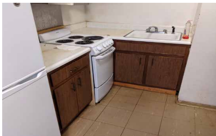
50-year-old kitchen with failing systems at the Campello Highrise.
