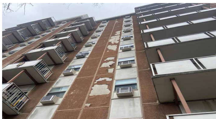
The granular façade surface and waterproofing coating have failed.
